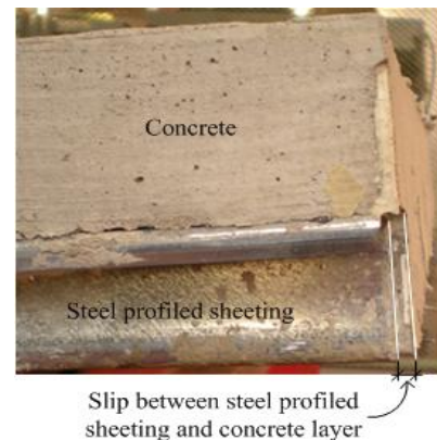
Fig 11. Slip between the layers in a composite steel – concrete slab
